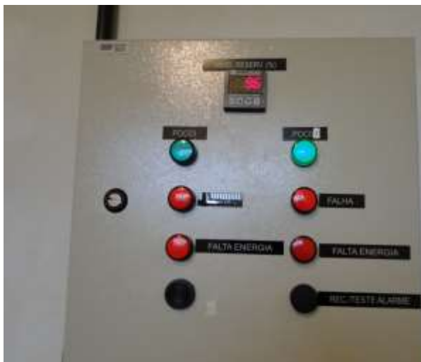
Painel de controle
